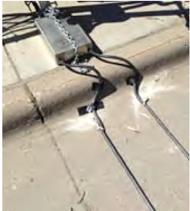
Figure A-4. Pneumatic Tube Installation
